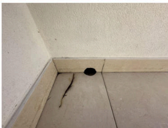
Fig. 6.1c — Drainage outlet at the wall, partly blocked with debris.
