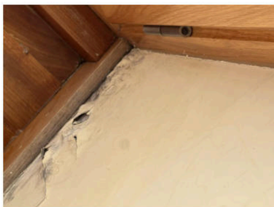
Fig. 6.3a — Window reveal: blistered and split lime finish along the timber lining.
