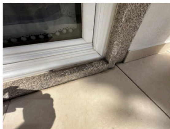
Fig. 6.1d — Frame and granite sill junction onto the veranda; seal aged and gapped.
