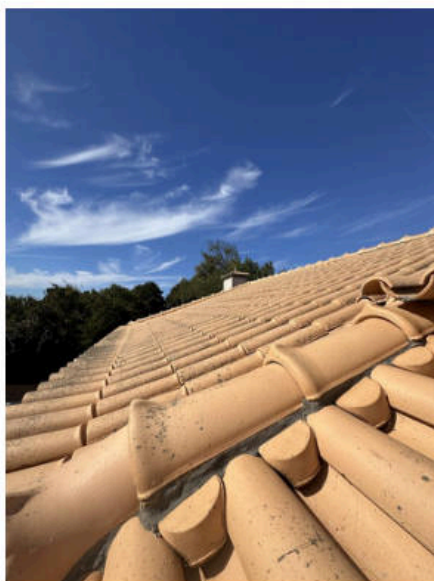
Fig. 6.5a — Ridge tiles: weathered and cracked bedding mortar, lichen on the tiles.
