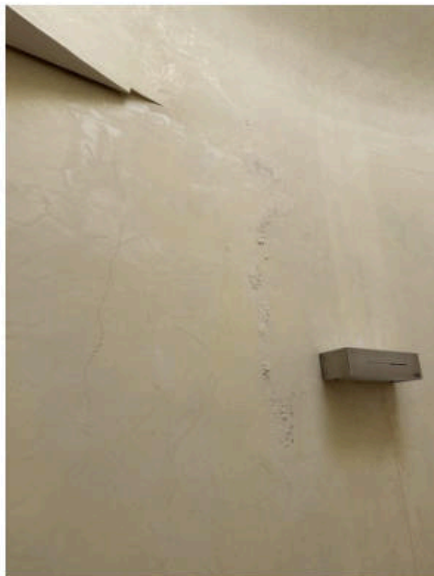
Fig. 6.4a — Inside the stair tower: vertical line of blistering with white salts in the lime finish.
