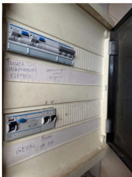
Fig. 8a — Garage board: the three-phase car charging circuit.
