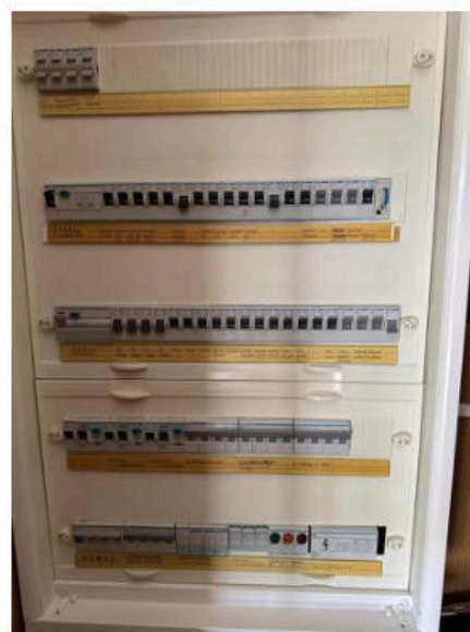
Fig. 8b — Main distribution board: labelled circuits with RCD protection.
