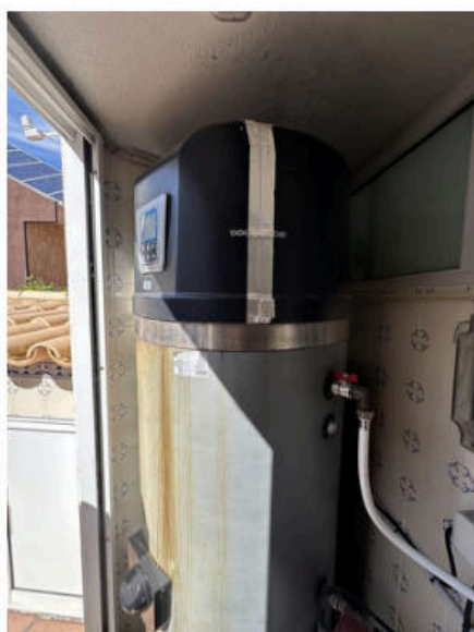
Fig. 6.7a — Heat-pump hot water cylinder: rust streaks down the casing.
